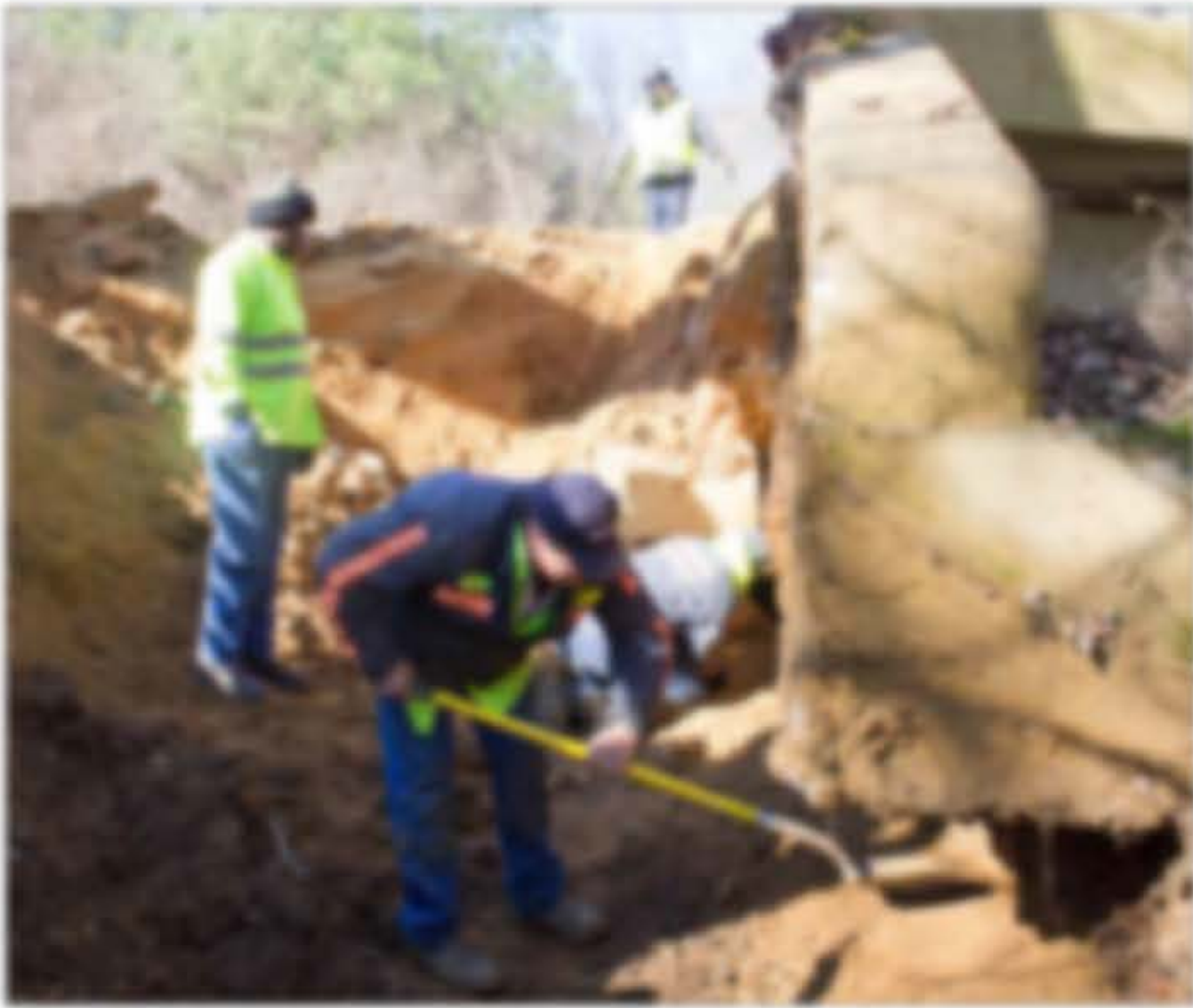
Oktibbeha County road workers Mark Young (middle) and Tom Hensley (right) are working on the main concrete structure of a bridge on New Creek Road in north Oktibbeha County near the Clay County line. Road work, including repair of the bridge, began in August and is expected to be completed by the end of the year. (Photo by Alan Wells)
